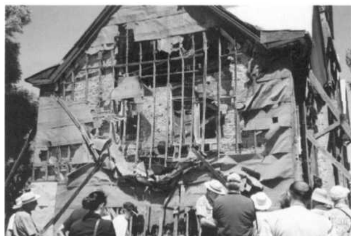
Restoration is underway on the south wall. Reinforced steel rods "tie stone to stone and brick to brick". Photo by Suzanne Everett.
