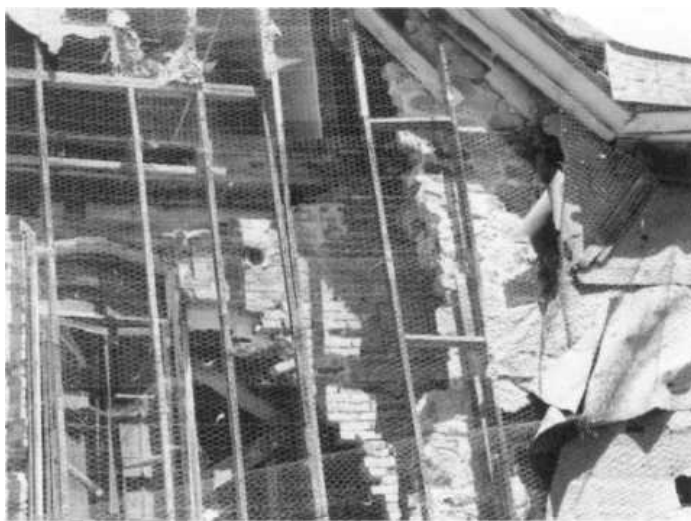
Close up of brick and stone work in progress on south wall.
