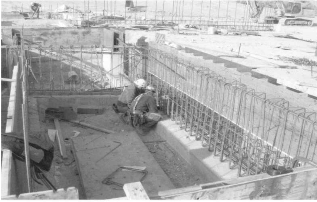
Don Ponciano (left) & Josh Triner (right) tie in rebar on an exterior wall ...creating a "cage" of reinforcement for the concrete wall.
